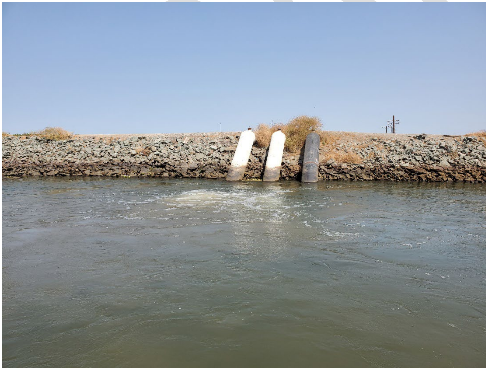
Figure 25. Agricultural drain water being pumped into the waterway near NORT-018
