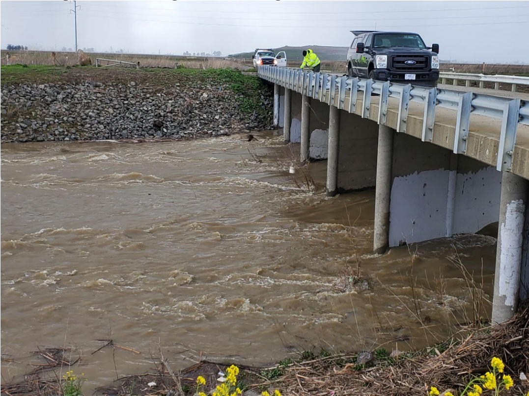
Figure A.19. High flow sampling from the bridge at Ulatis Creek, February 28, 2023.
